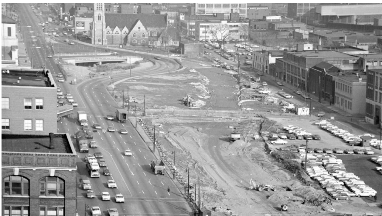
Detroit Hasting Street under demolition to build Chrysler and Fisher Freeways in the early 1960s (Source: Abayomi Azikiwe)
