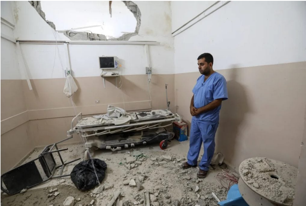
Dr Suleiman Qaoud surveys the damage at the Rantisi Specialist Hospital, part of the Nasser Medical Complex in Gaza City, following Israeli missile attacks on November 6, 2023 [Abdelhakim Abu Riash/Al Jazeera]
