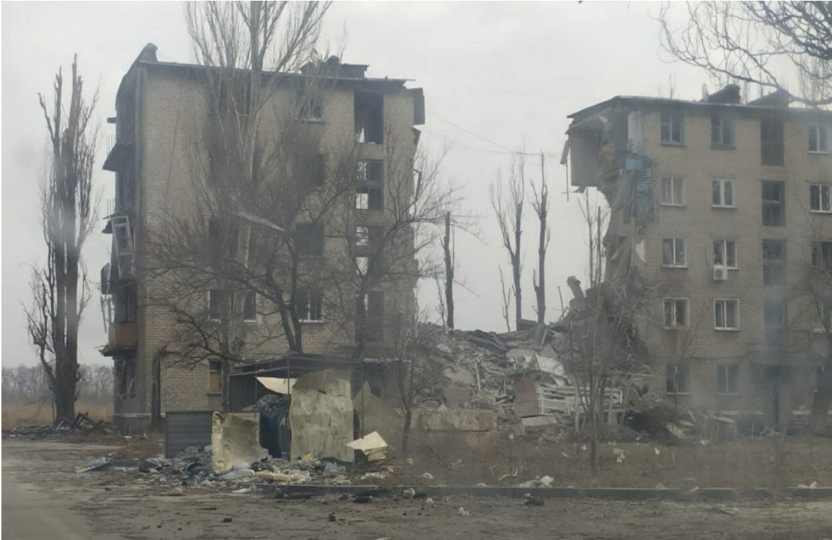
Residential building in Avdiivka city (Donetsk region of Ukraine) after Russian shelling and airstrikes on the city on 17 March 2023 (Licensed under CC BY 4.0)
