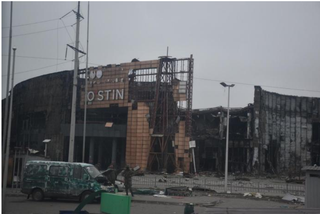
A destroyed shopping mall in the city center [Source: Photo courtesy of Sonja van den Ende]
