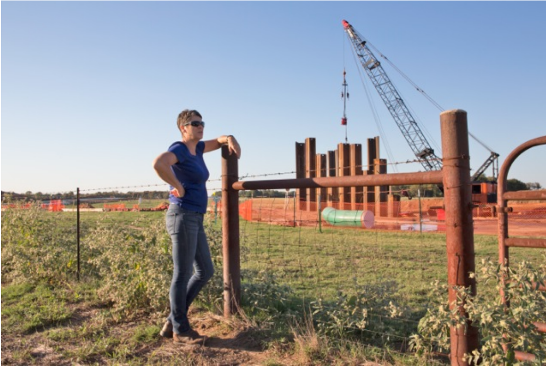
Julia Trigg Crawford peers into a TransCanada construction site adjacent to her land ©2012 Julie Dermansky
