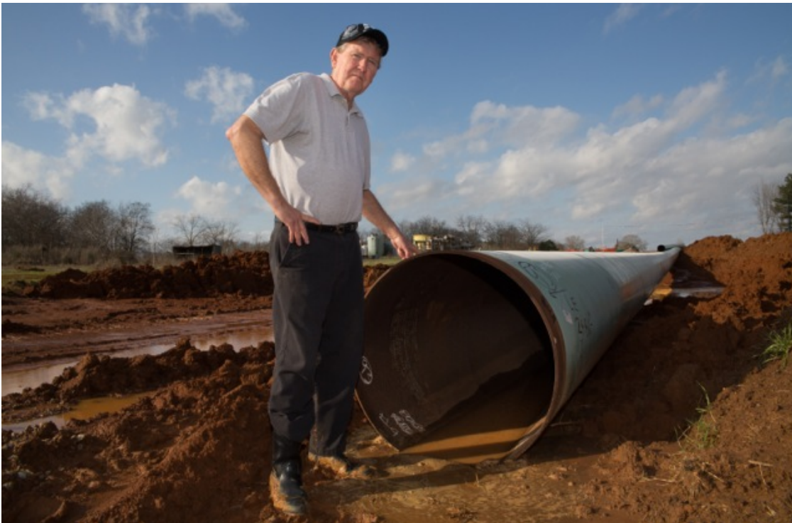
Michael Bishop stands in front of a section of the Keystone XL pipeline before it was installed on his property. ©2013 Julie Dermansky
