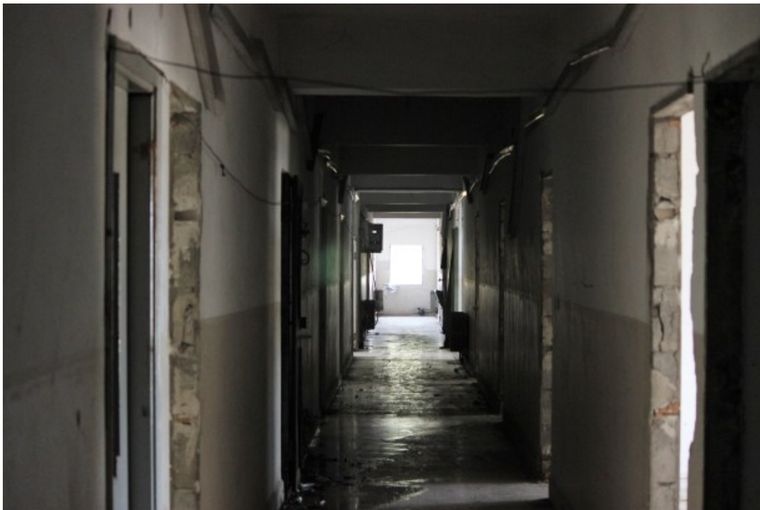
The entire RSCD building had been converted into a military outpost with all rooms sandbagged and windows turned into sniping points. (Photo: Vanessa Beeley)
