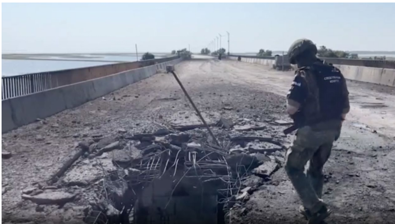
The Chonhar Bridge following an attack using French-made SCALP missiles, August 2023
