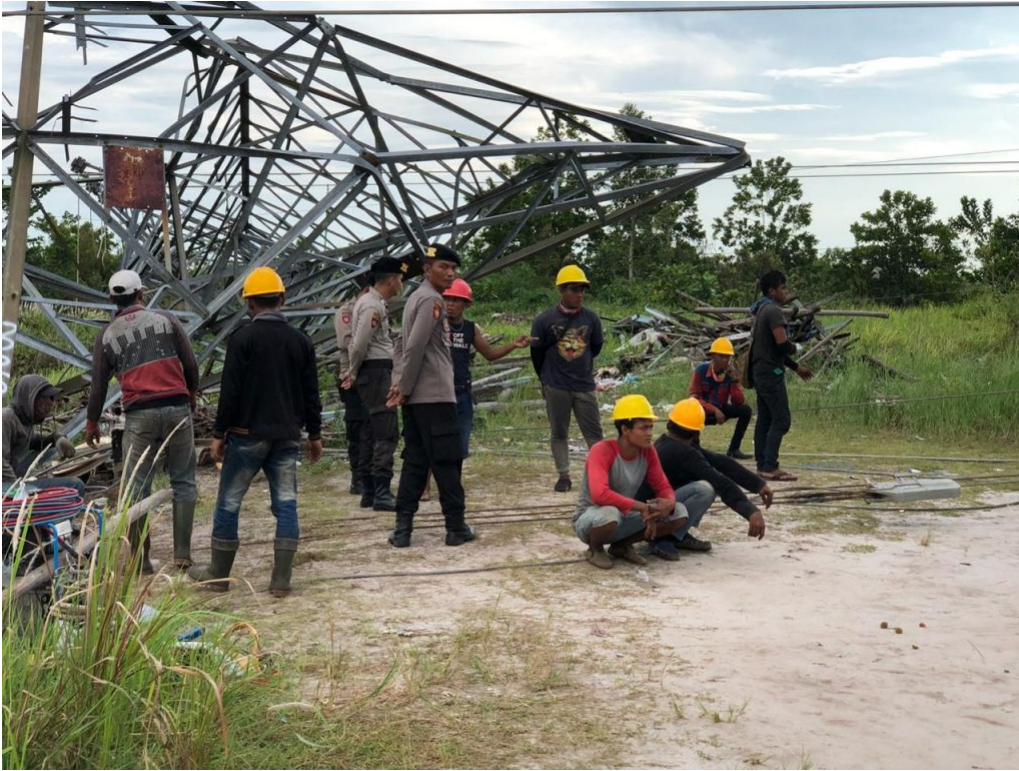
Collapsed high voltage tower near Palangkaraya
