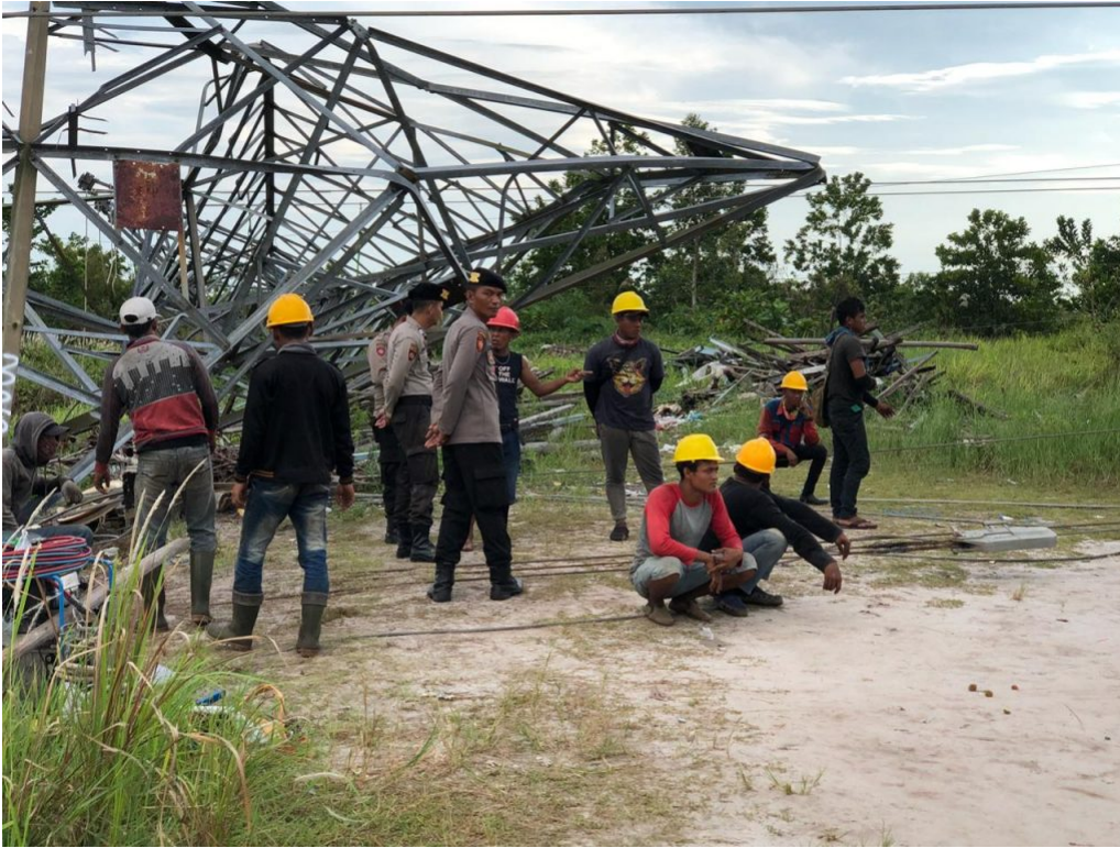
Collapsed high voltage tower near Palangkaraya
