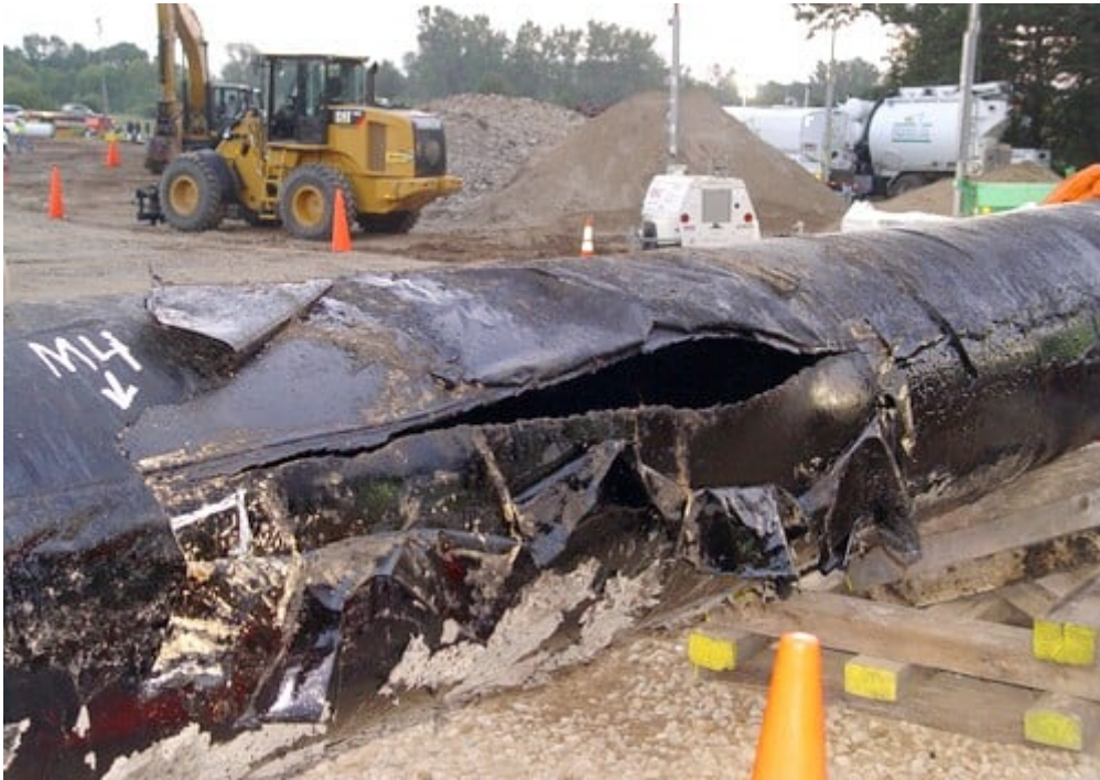
The Enbridge pipeline rupture that contaminated the Kalamazoo River on July 25, 2010
