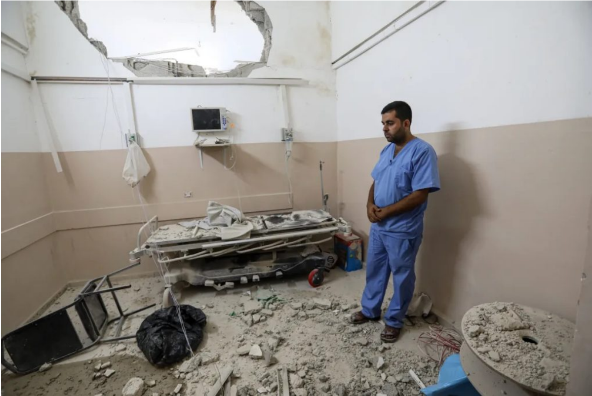
Dr Suleiman Qaoud surveys the damage at the Rantisi Specialist Hospital, part of the Nasser Medical Complex in Gaza City, following Israeli missile attacks on November 6, 2023 [Abdelhakim Abu Riash/Al Jazeera]
