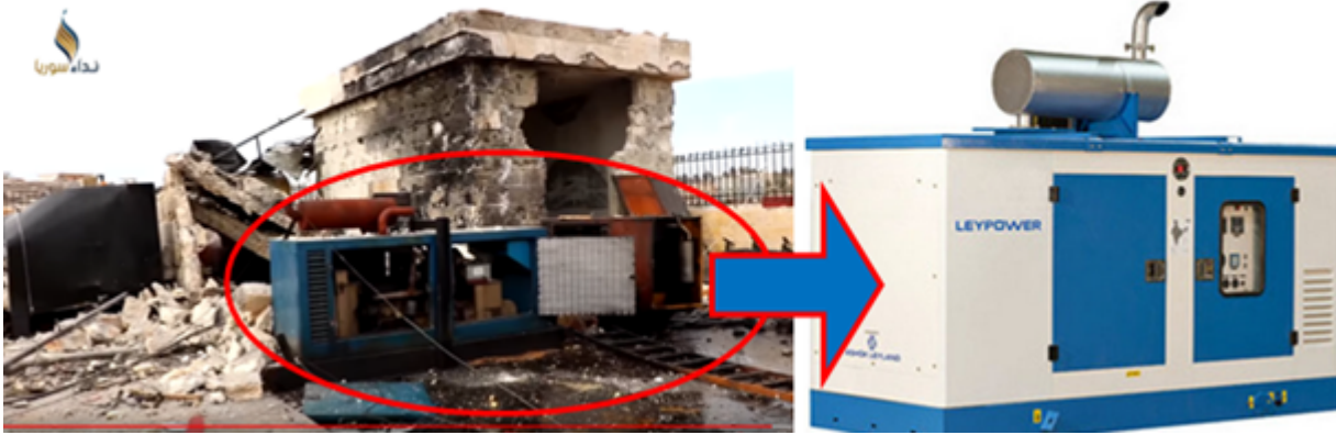
Diesel generator destroyed by fire dated March 25, 2017.
