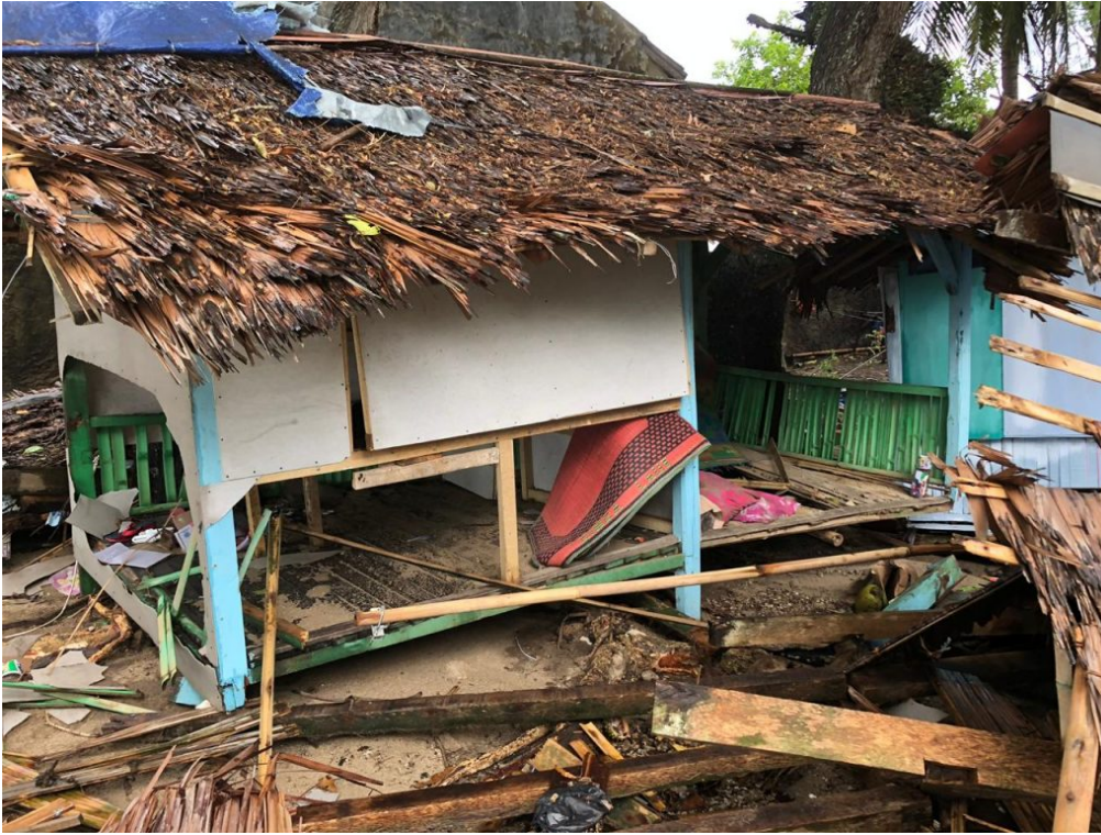
Miserable structures could not withstand tidal wave
