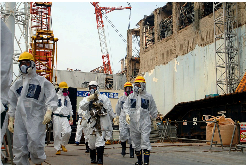
IAEA Experts at Fukushima Daiichi Nuclear Power Plant Unit 4, 2013 (Source: Wikimedia Commons )
