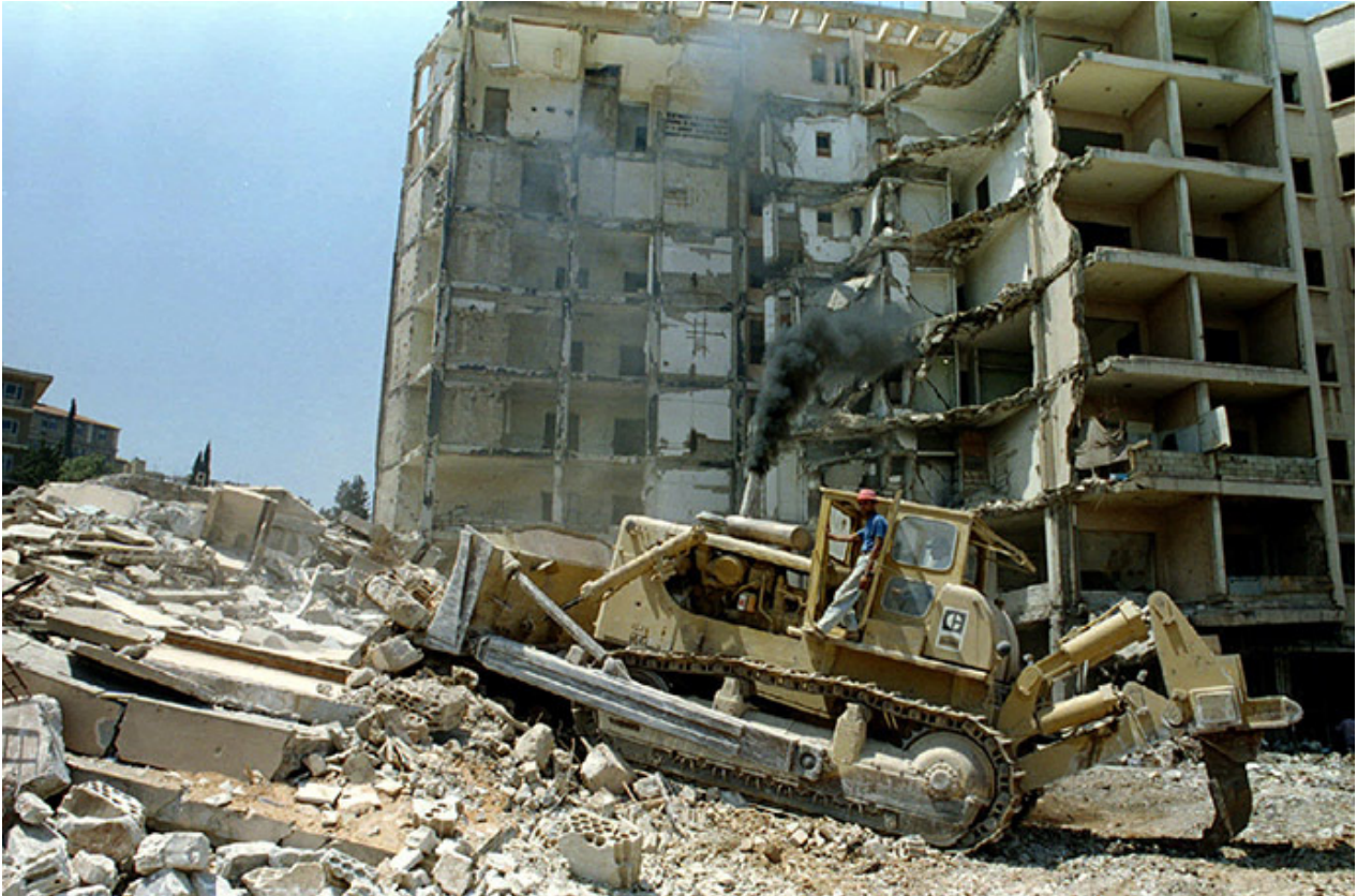
FILE PHOTO: A bulldozer demolishes the bombed out building of the American embassy in Beirut. (Reuters)
