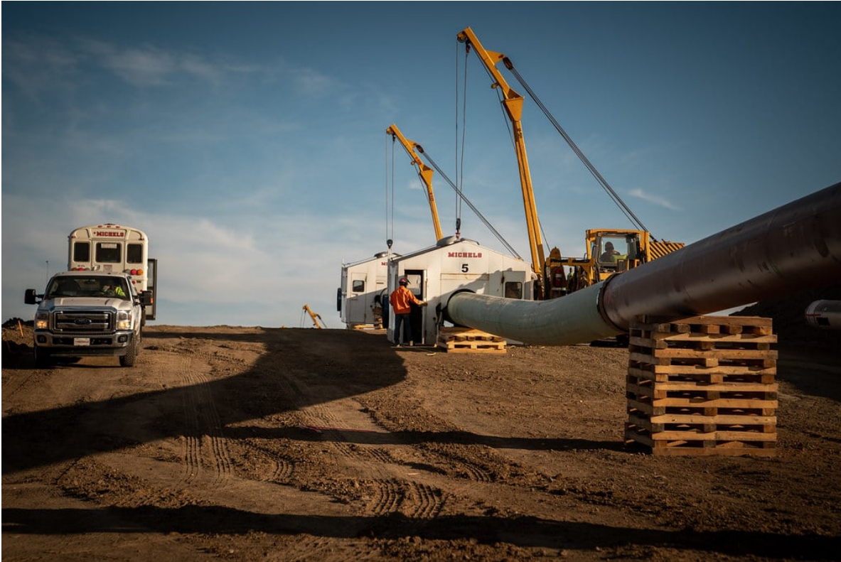
Construction of Keystone XL in Oyen, Alberta. October 2020. Credit: Government of Alberta . CC BY-NC-ND 2.0
