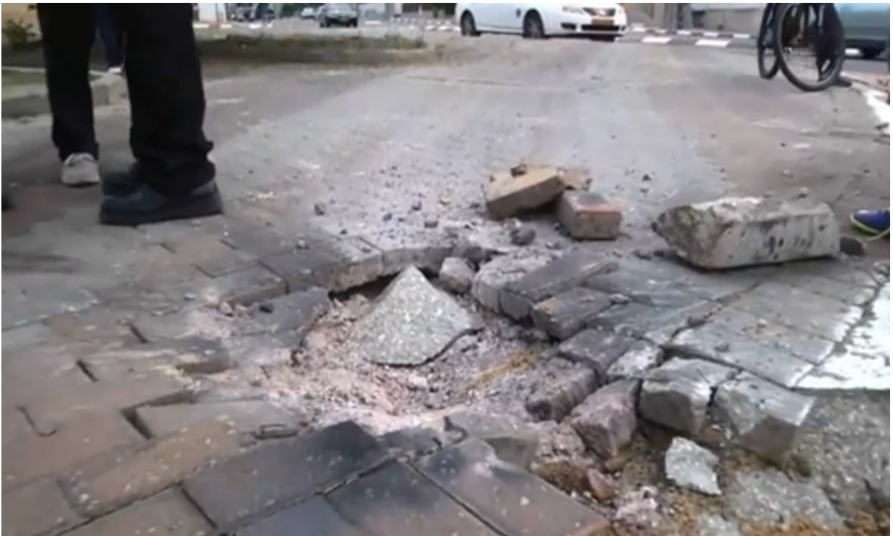
Damage caused in Gaza by Israeli projectiles:
