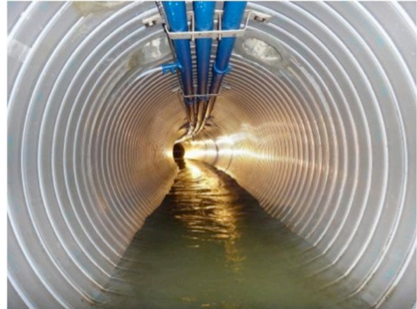
Sendai's Heat-Recovery Sewerage Test
